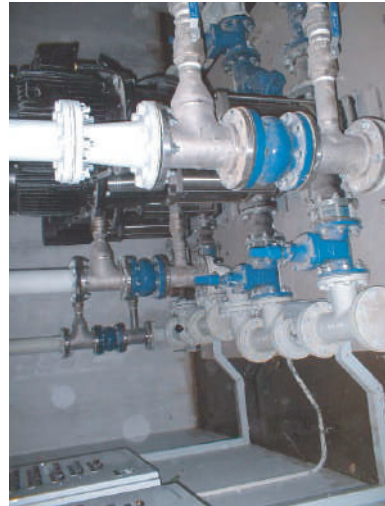
Side view of pump room.
